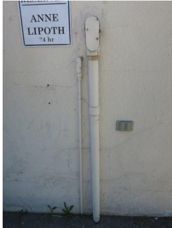
Photo 14 - Holes in Stucco not Sealed
