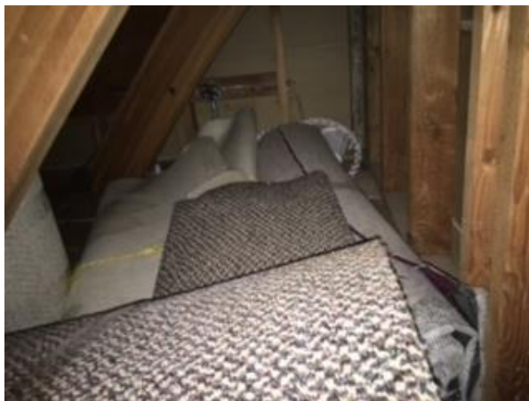
Photo 47 - Arches on Left, Room Framing on the Right in the Room over Main Floor Chair Storage Room
