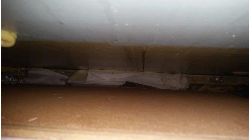
Photo 98 - Looking Down on Kitchen Material on Top of Hot Water Heating Radiators
