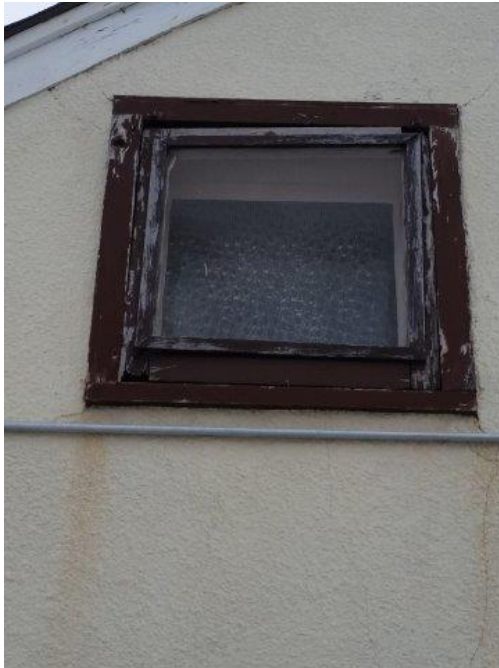
Photo 19 - Window in North wall of Upper Bedroom (now office) with Rotted Frame
