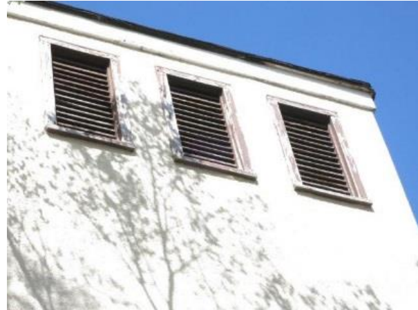
Photo 41 - Louvres on Faux Bell Tower
