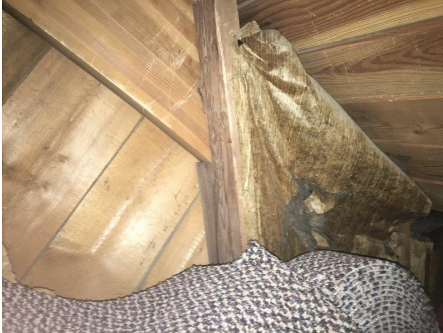
Photo 49 - South Wall Framing Composed of arch, Timber Framing and Diagonal Shiplap Lumber. Note Lack of Insulation on Portions of the Wall.
