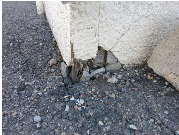
Photo 18 - Damage to Hall Corner. Note Wall is Below Surface at this Location
