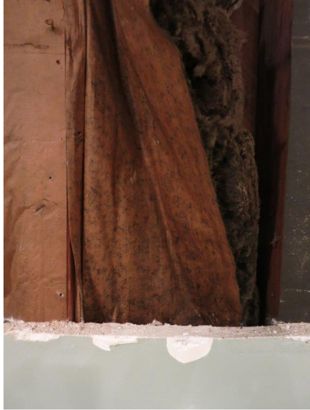
Photo 65 - Mould on Paper-Backed Insulation in Wall Cavity
