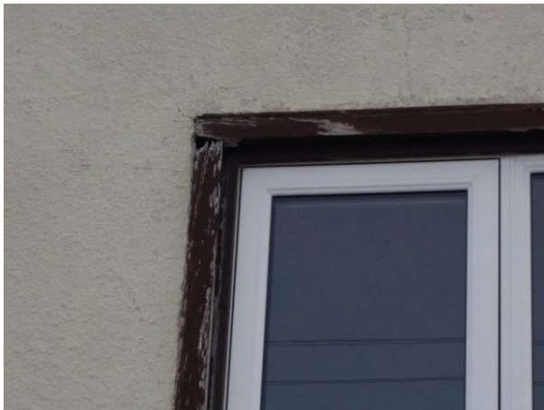
Photo 23 - Rotted Frames around Replacement Thermopane Sealed Window Units
