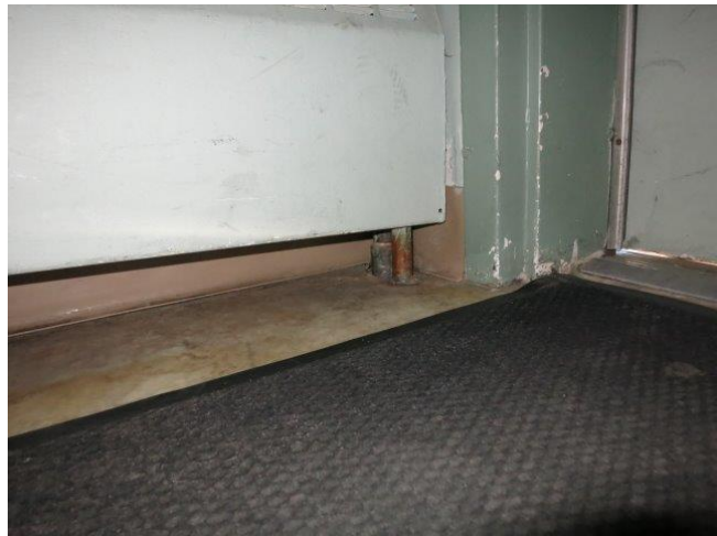
Photo 61 - Deteriorated Floor Covered with Matting; Note Light Under Left Edge of Door
