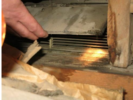
Photo 38 - Opening for Ventilation (Exit location is inside the Hall at the Stairway over the original entrance)
