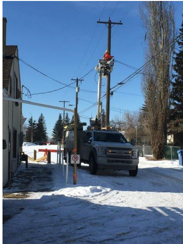
Photo 104 - Utility Required Fused Disconnect Switch to Allow their Linemen to Isolate the Hall Electrical Load from the Utility Supply
