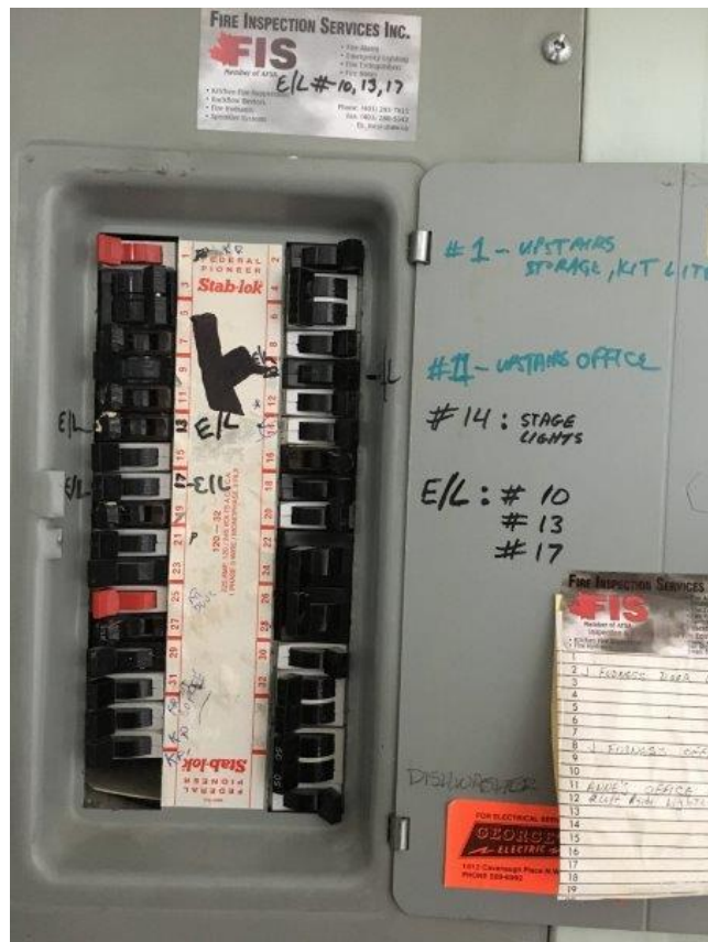
Photo 100 - Circuit Breaker Panel Supplying Hall from Church
