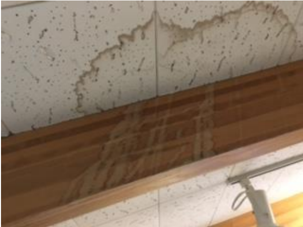
Photo 44 - Water Stains in Ceiling of Upstairs Office
