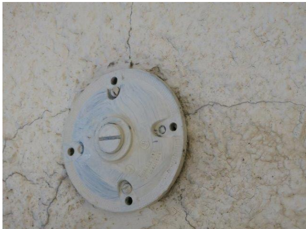
Photo 16 - Improperly Covered and Sealed Electrical Fittings
