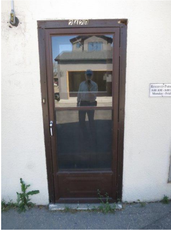
Photo 21 - North End door With very Rotted Frame
