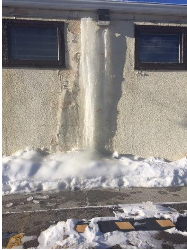
Photo 51 - Icicles along East Wall of Hall
