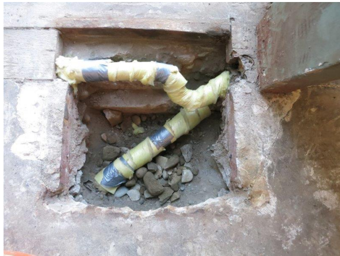
Photo 95 - Hot Water Heating Pipes at East Entrance Door. Insulation Added When Floor was Replaced in 2016 to Keep Pipes from Freezing Near Doorway
