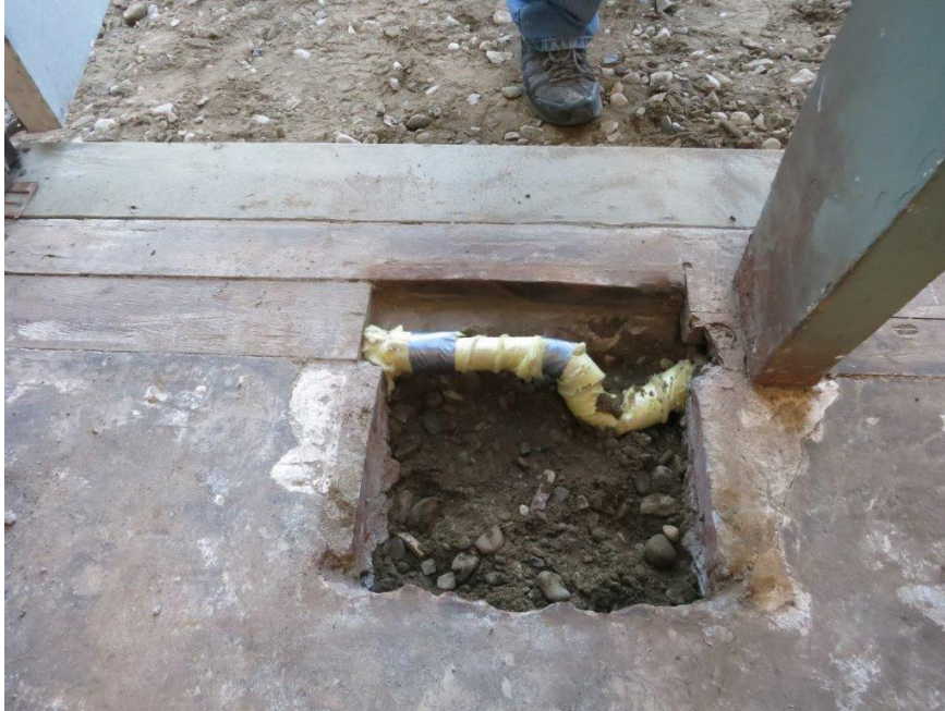
Photo 10 - Arch rib to edge of concrete slab on grade floor/foundation. (Note pipe has been insulated in this one location only)
