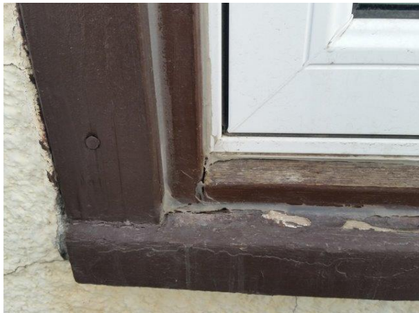
Photo 24 - Rotted Frames around Replacement Sealed Window Units
