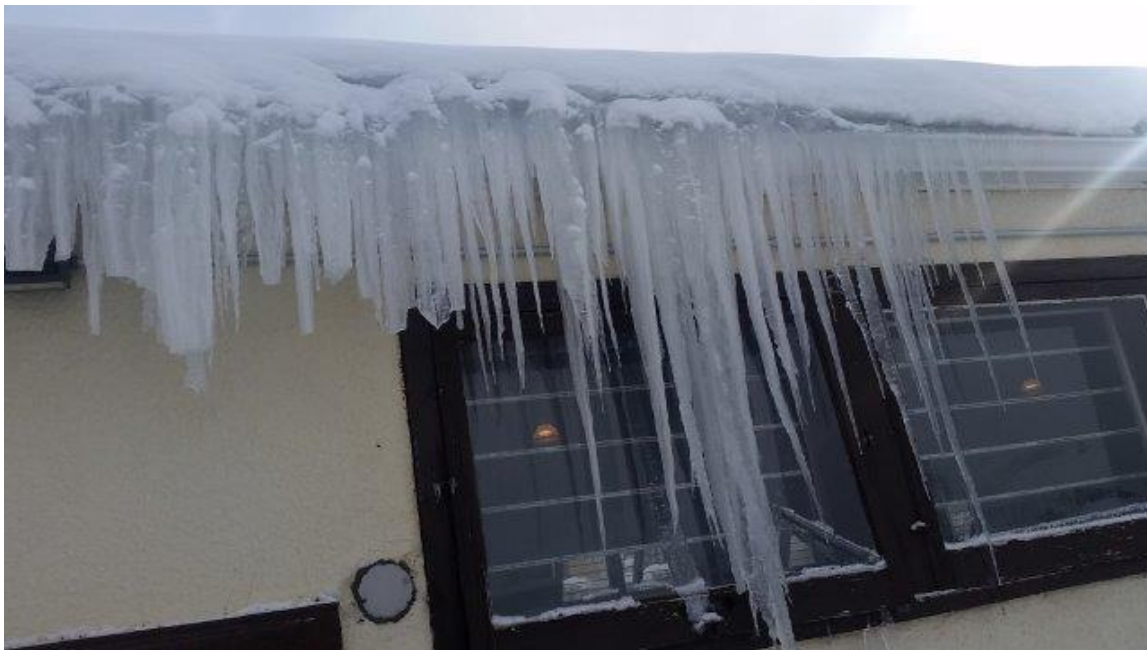
Photo 52 - Icicles along West Walls of Hall. Icicles from melted Snow on Poorly Insulated Roof
