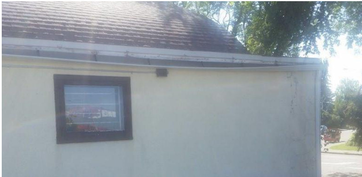
Photo 107 - Eaves Trough Damage from Ice Filling Eaves Trough
