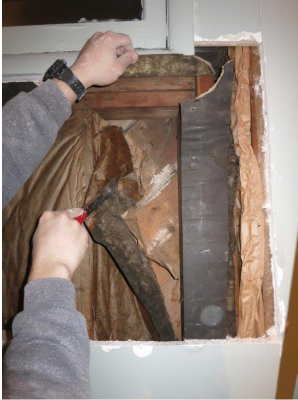
Photo 64 - Top right side of west wall under window. Minor damage on outside wood sheathing. Very incomplete vapour barrier. Tar paper over double framing members.
