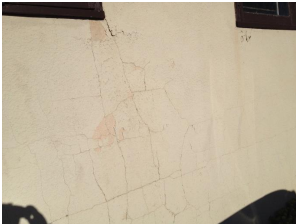
Photo 11 - Exterior of the Hall – Paint layer over stucco is falling off and cracks are forming in stucco
