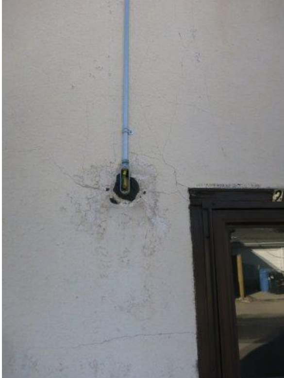
Photo 13 - Open Electrical Conduit Penetration through the Stucco Wall
