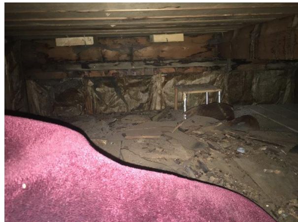
Photo 48 - Top of West Wall (at back of photo); Underside of Flat Portion of Roof (at top of photo); Water Leakage and Re-Roofing Debris in Foreground
