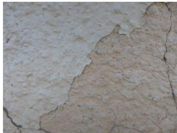
Photo 12 - Peeling Paint and Cracks in Underlying Stucco
