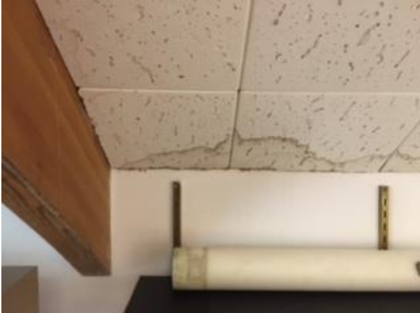
Photo 45 - Water Stains in Ceiling of Upstairs Office
