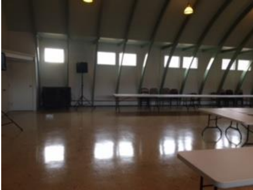
Photo 78 - West side Wall of Main Hall showing Arch Ribs, Windows, and Relocatable Stacking Tables and Chairs
