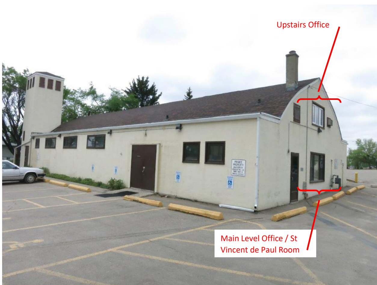
Photo 75 – View of Hall from NE Corner of the Hall (showing upper and lower meeting/office rooms)
