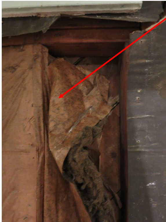
Photo 62 - Wall Insulation that is Sagging, Unsupported and Incompletely Covering Wall
