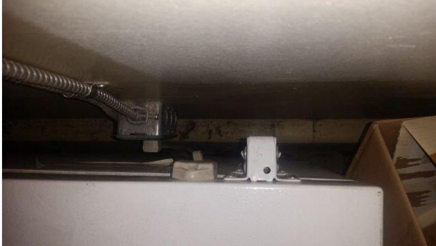
Photo 96 – Looking Down on Deep Freeze Blocking Hot Water Heating in Janitorial Storage Room
