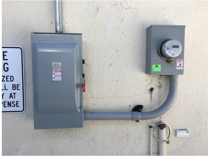
Photo 101 - New (2020) Independent Electrical Supply from Utility
