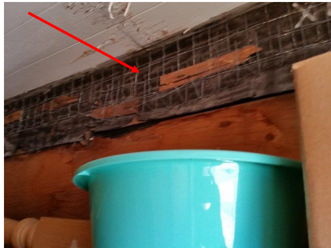
Photo 32 - Unfinished Exterior Wall Where Original Entrance Vestibule was Located
