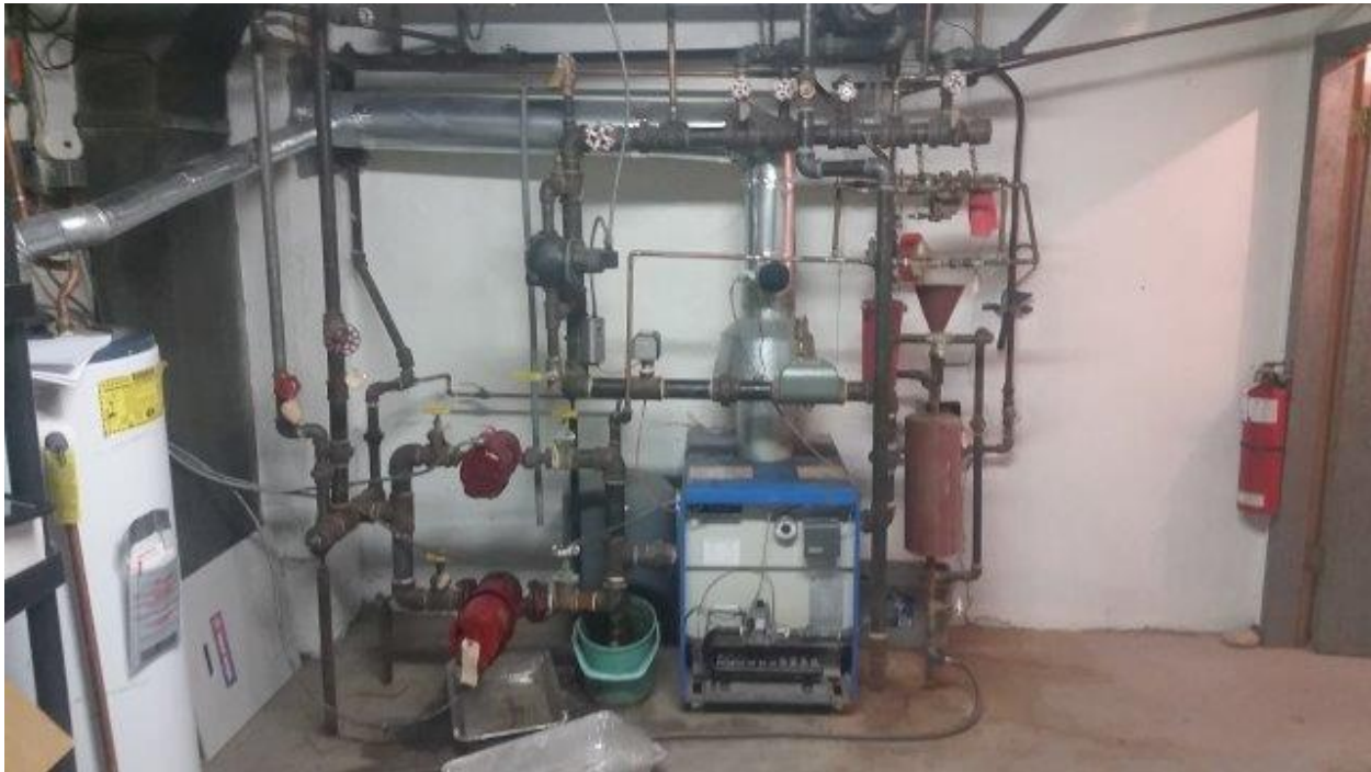
Photo 87 - Hot Water Heating Boiler in Hall Basement
