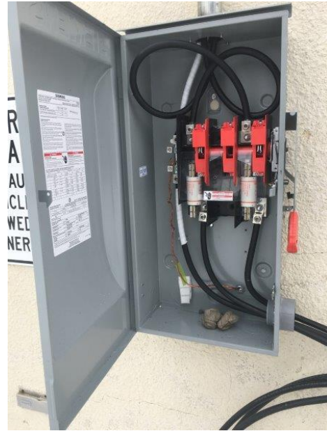
Photo 102 - Fused (200 A) Disconnect Switch to Isolate Hall Electrical Load from Utility
