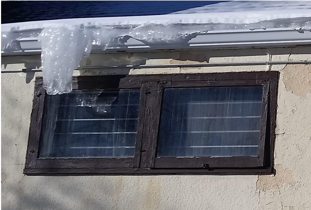
Photo 53 - Icicles along West Walls of Hall. Icicles from melted Snow on Poorly Insulated Roof. Note Window that will Not Close.
