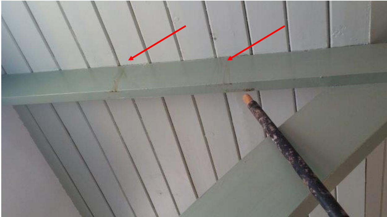
Photo 42 - Water Leakage on the Interior/Underside of the Roof
