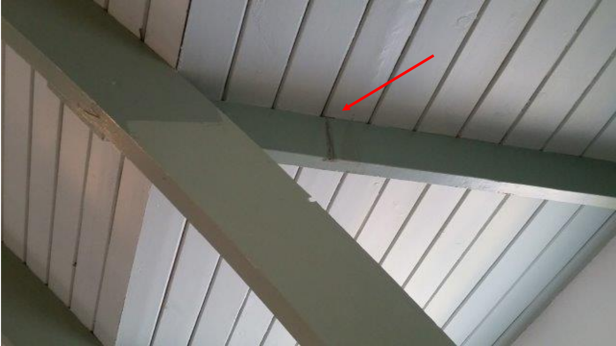
Photo 43 - Water Leakage on the Interior/Underside of the Roof
