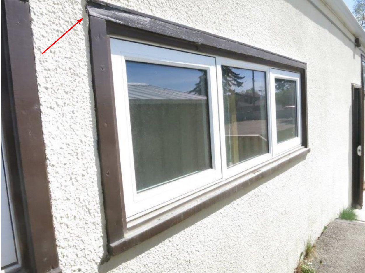
Photo 25 - New Sealed Double Glazed Windows set into Original Frames that are now Rotting. Note how this West Wall of the Hall is Buried Under the Asphalt
