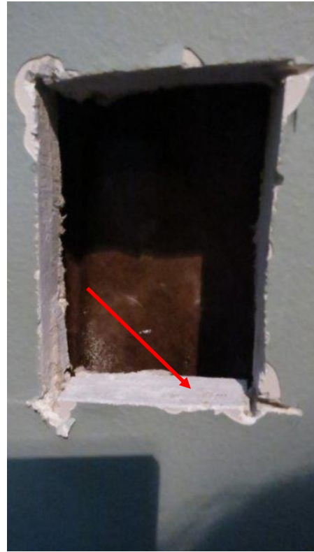
Photo 55 - Hole on Inside Hall Wall where Sample was Taken for Hazardous Material Sampling. Note line between Hardboard and Drywall Materials
