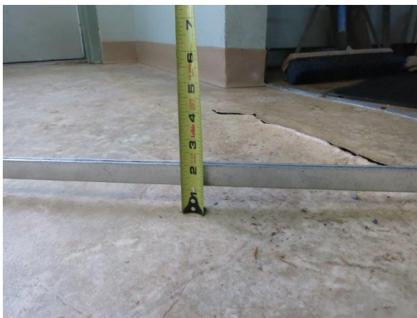
Photo 56 - Sagging floor at main entrance to hall
