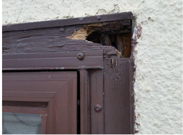
Photo 22 - North Door Frame Rot
