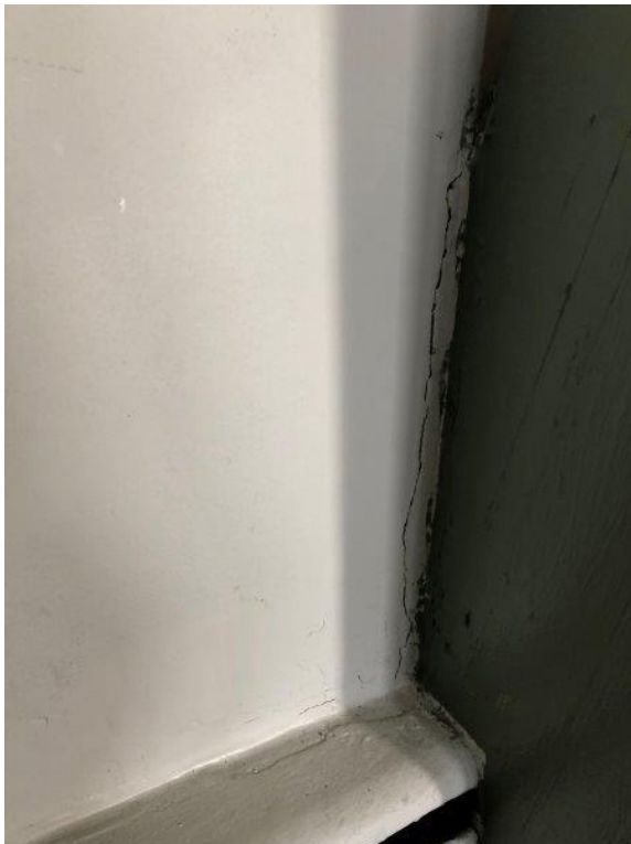
Photo 8 - Arch to Interior Wall Seam Cracking
