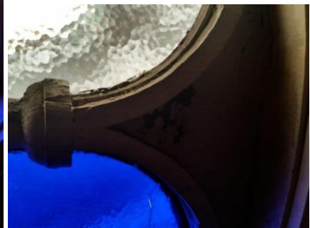
Photo 28 - Rotted Wood in Hand Built Stained Glass Window
