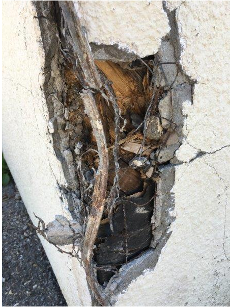
Photo 15 - Damage to Corner of Hall Interior Wall Wood Exposed to Water
