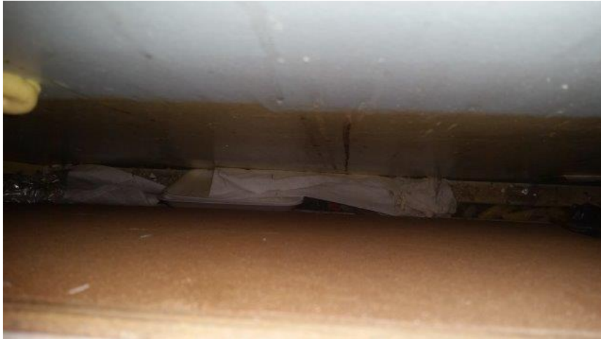
Photo 86 - Looking Down on Kitchen Material on Top of Hot Water Heating Radiators
