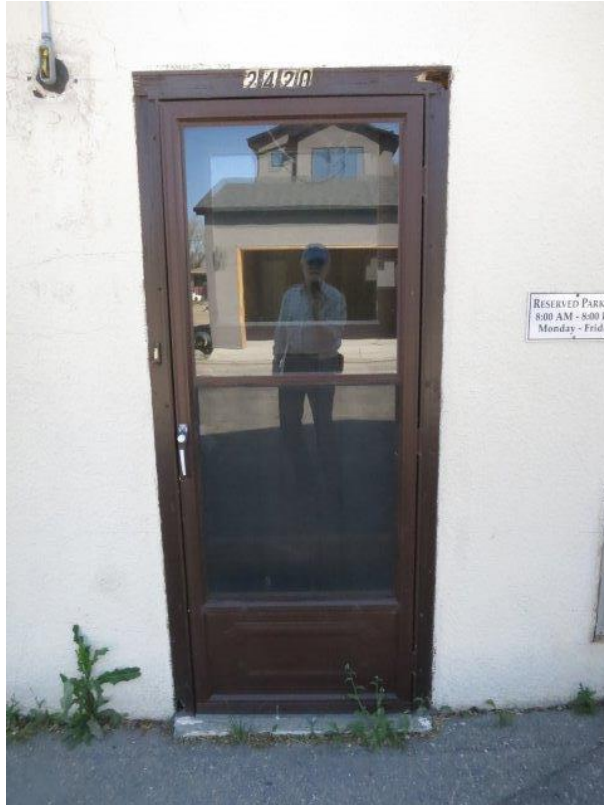
Photo 19 - North End door With very Rotted Frame
