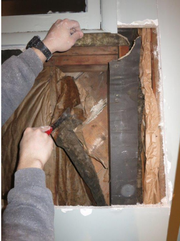
Photo 56 - Top right side of west wall under window. Minor damage on outside wood sheathing. Very incomplete vapour barrier. Tar paper over double framing members.
