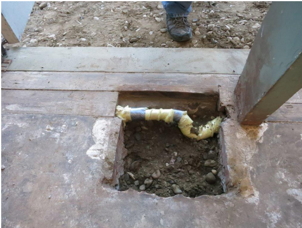
Photo 8 - Arch rib to edge of concrete slab on grade floor/foundation. (Note pipe has been insulated in this one location only)
