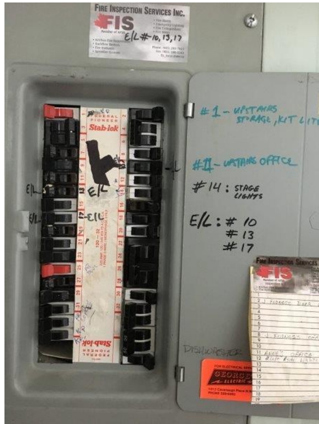
Photo 88 - Circuit Breaker Panel Supplying Hall from Church
