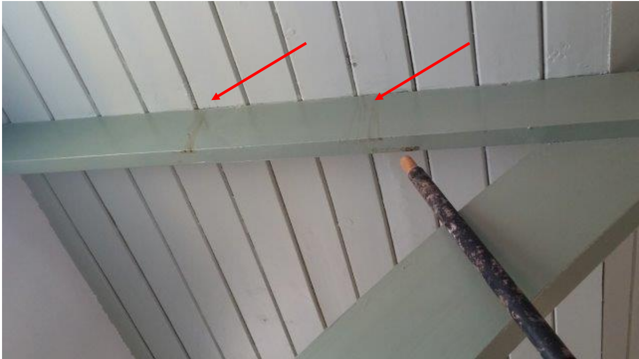
Photo 40 - Water Leakage on the Interior/Underside of the Roof
