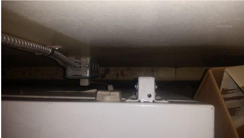
Photo 84 – Looking Down on Deep Freeze Blocking Hot Water Heating in Janitorial Storage Room
