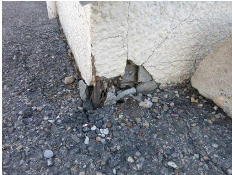
Photo 16 - Damage to Hall Corner. Note Wall is Below Surface at this Location
