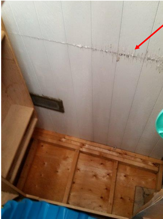
Photo 29 - Leaking Roof in Church Original Entrance Vestibule
