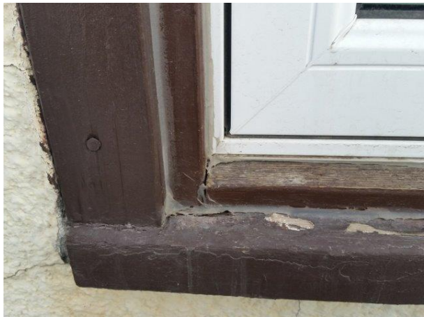
Photo 22 - Rotted Frames around Replacement Sealed Window Units
