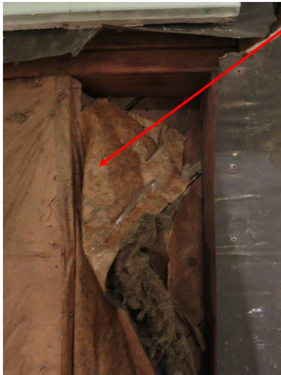
Photo 54 - Wall Insulation that is Sagging, Unsupported and Incompletely Covering Wall
