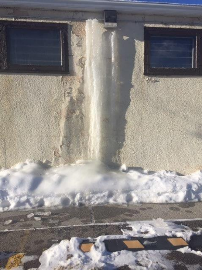
Photo 43 - Icicles along East Wall of Hall
