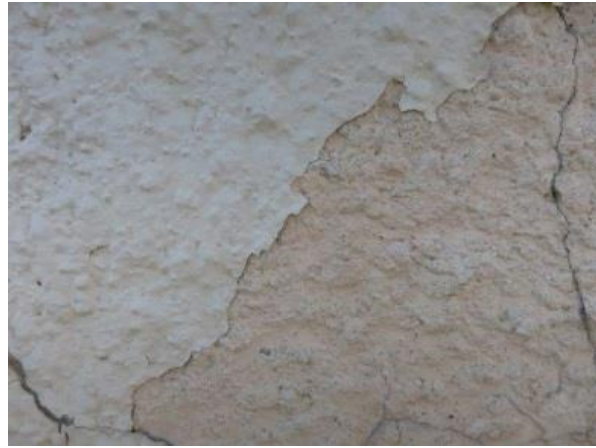
Photo 10 - Peeling Paint and Cracks in Underlying Stucco
