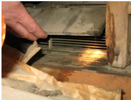
Photo 36 - Opening for Ventilation (Exit location inside hall is unknown)
