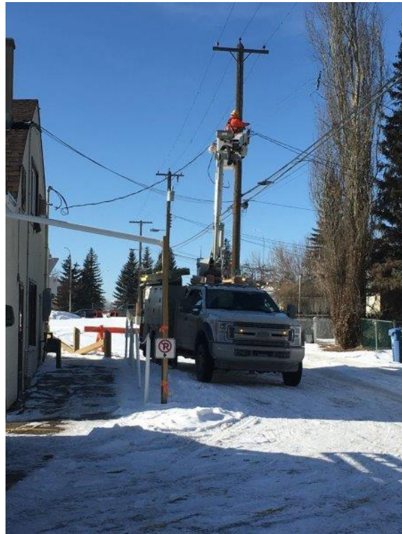
Photo 92 - Utility Required Fused Disconnect Switch to Allow their Linemen to Isolate the Hall Electrical Load from the Utility Supply
