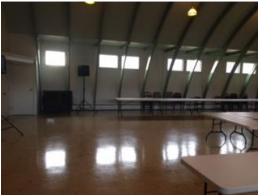
Photo 70 - West side Wall of Main Hall showing Arch Ribs, Windows, and Relocatable Stacking Tables and Chairs
