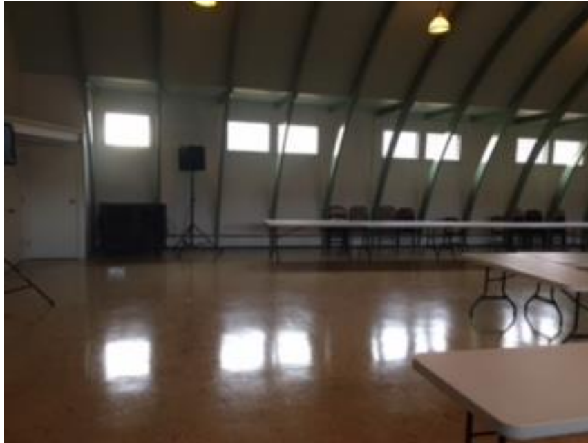
Photo 7 - Arch Rib Construction along the Straight Walls Intrude into Main Hall Space
