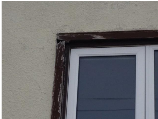
Photo 21 - Rotted Frames around Replacement Thermopane Sealed Window Units
