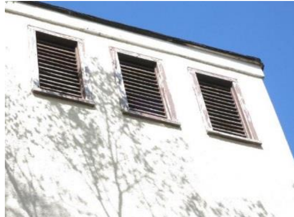
Photo 39 - Louvres on Faux Bell Tower
