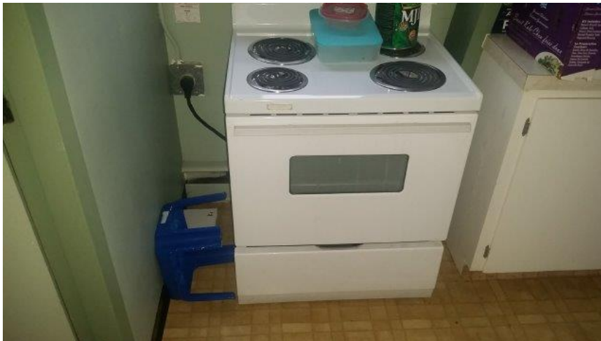
Photo 85 - Kitchen Appliances and Cupboards Blocking Hot Water Heating Radiators
