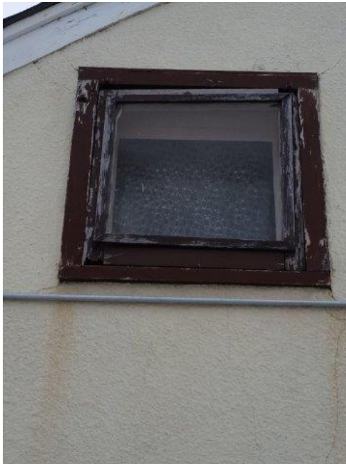
Photo 17 - Window in North wall of Upper Bedroom (now office) with Rotted Frame
