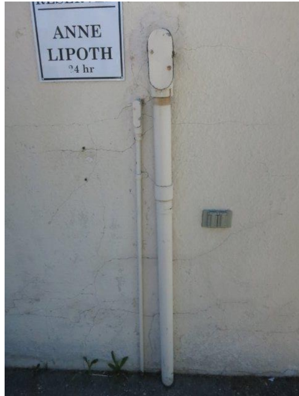
Photo 12 - Holes in Stucco not Sealed
