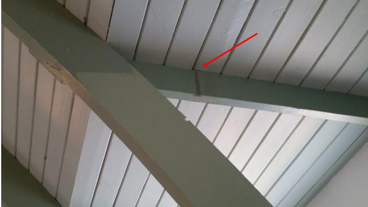
Photo 41 - Water Leakage on the Interior/Underside of the Roof
