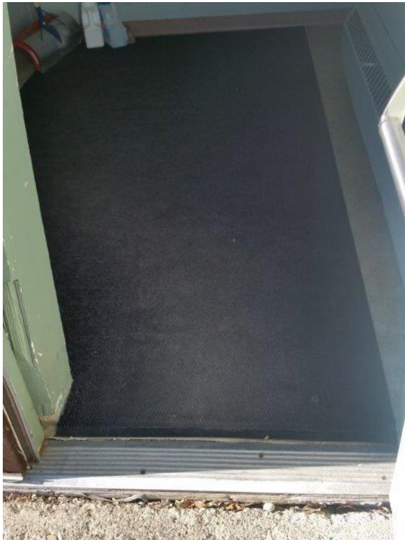
Photo 52 - Damaged Door Sill, Subsiding Door Ramp
