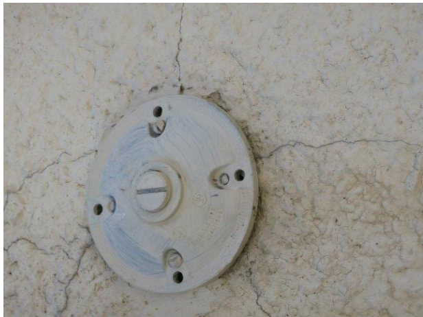
Photo 14 - Improperly Covered and Sealed Electrical Fittings
