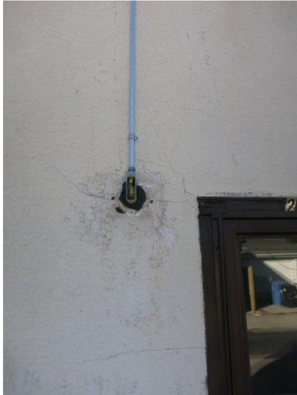
Photo 11 - Open Electrical Conduit Penetration through the Stucco Wall
