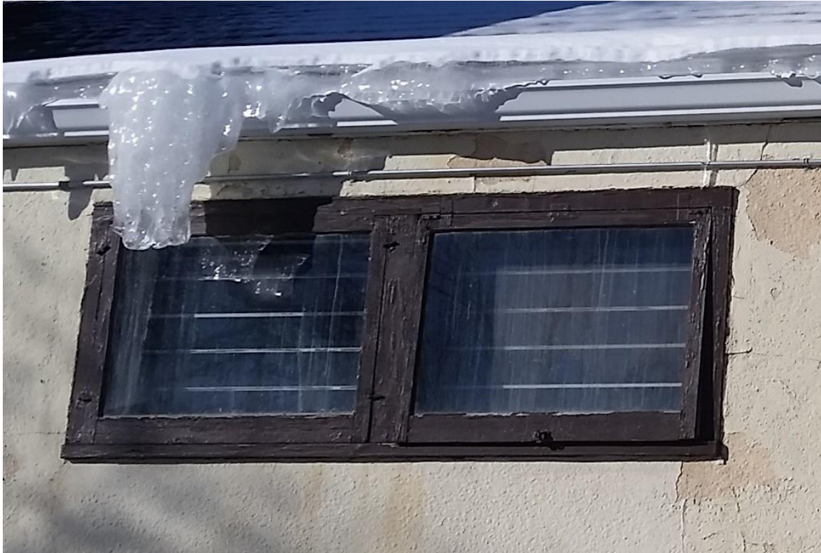
Photo 45 - Icicles along West Walls of Hall. Icicles from melted Snow on Poorly Insulated Roof. Note Window that will Not Close.
