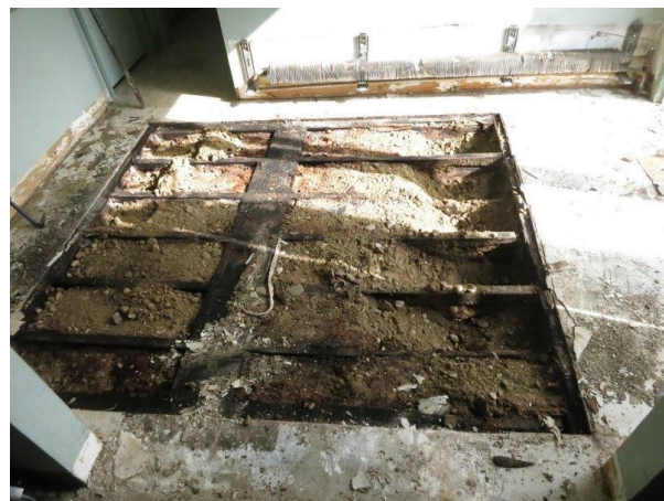
Photo 49 - Rotted Framing Below Main Entrance Floor
