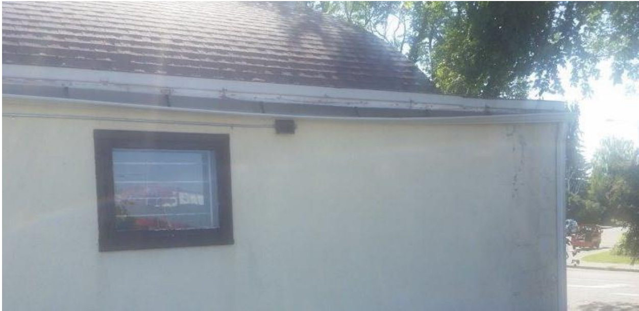
Photo 95 - Eaves trough Damage from Ice Filling Eaves Trough
