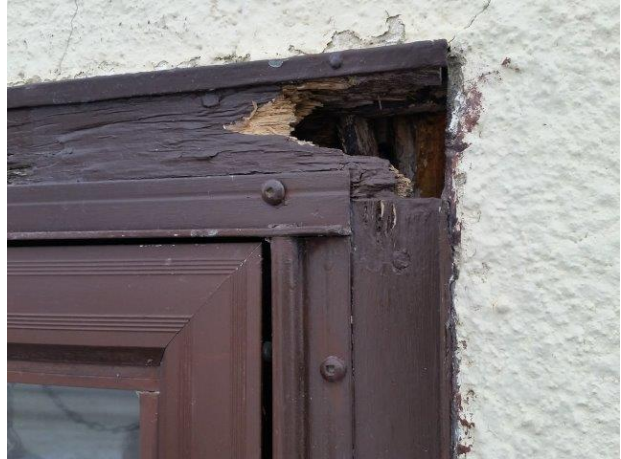
Photo 20 - North Door Frame Rot
