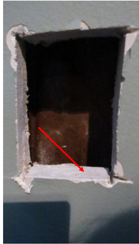
Photo 47 - Hole on Inside Hall Wall where Sample was Taken for Hazardous Material Sampling. Note line between Hardboard and Drywall Materials
