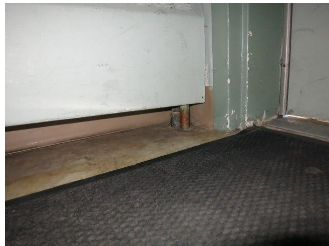
Photo 53 - Deteriorated Floor Covered with Matting; Note Light Under Left Edge of Door
