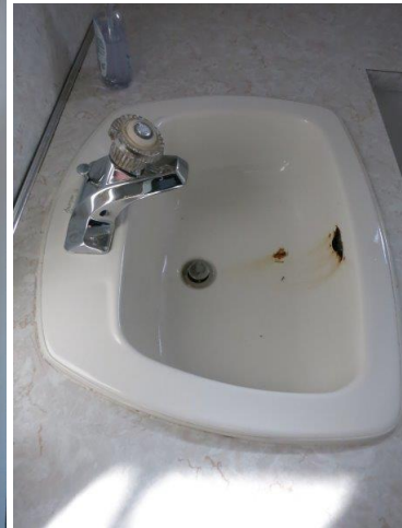
Photo 75 - Deteriorating Fixtures in Women's Washroom
