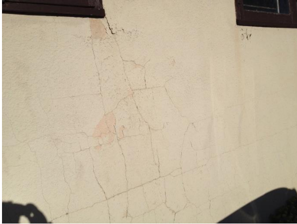
Photo 9 - Exterior of the Hall – Paint layer over stucco is falling off and cracks are forming in stucco
